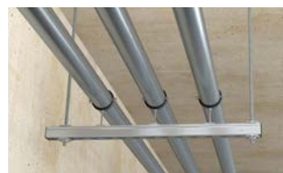
Pipe route on suspended channel: FAW
